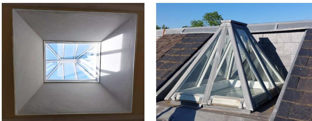
Figure 4: Cupola above a stair well with additional double glazing unit seen from below and above
