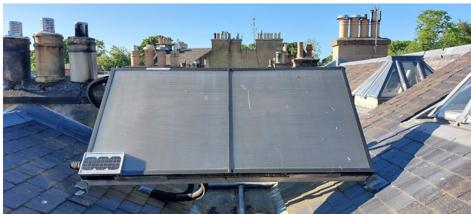
Figure 6: Water heating solar panel installed in roof valley
