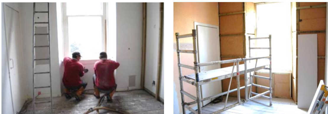
Figure 5: Injecting polystyrene insulation behind wall lining + Hemp board insulation between timber framing
